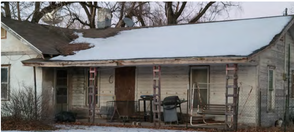
House in rural Reno County community needing siding, roof and porch repair
