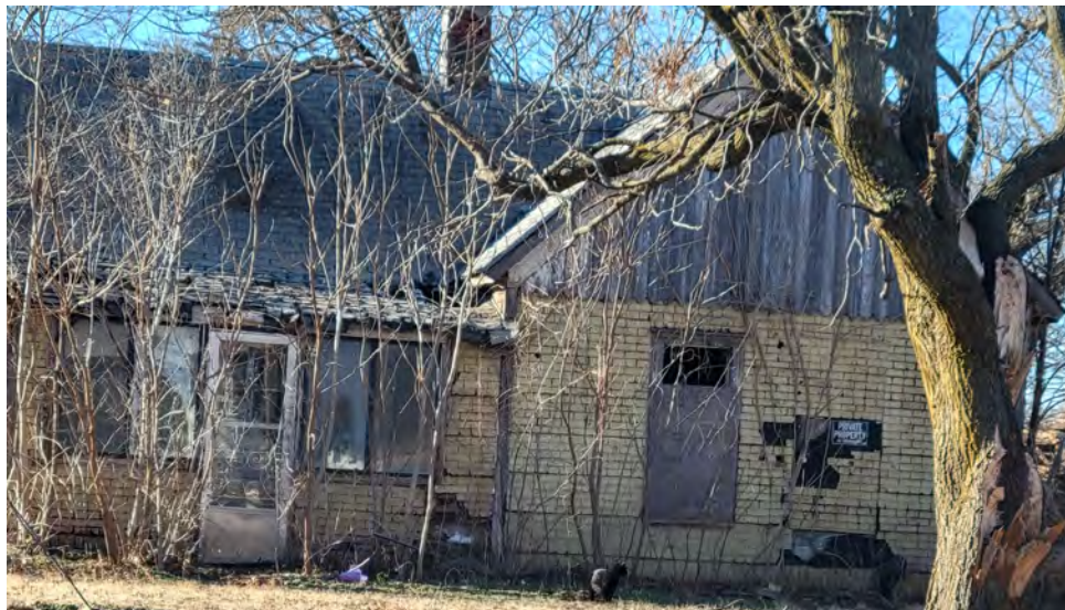
House in rural Reno County community needing demolished
